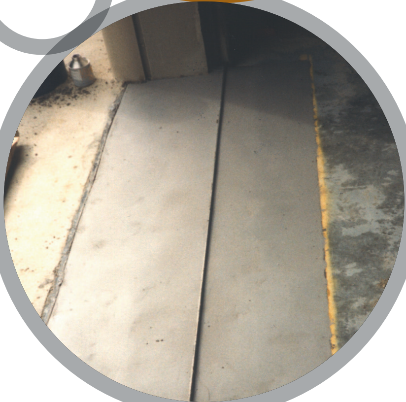
Floor Problem Areas
